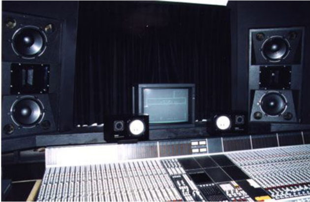
Soffited system, finished in flat black textured paint. Single woofer each side (not shown) As installed in the private studio of Dr. Dré
